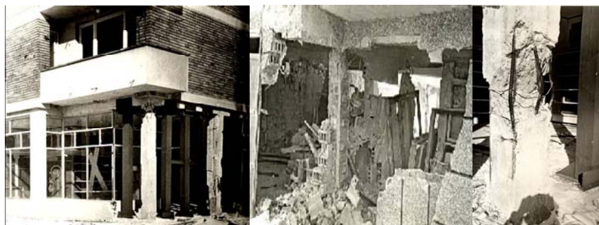
Figure 6: Block of Flats in Strazhitza (1986) – “Flexible” First Floor with Elements of Destructions.
